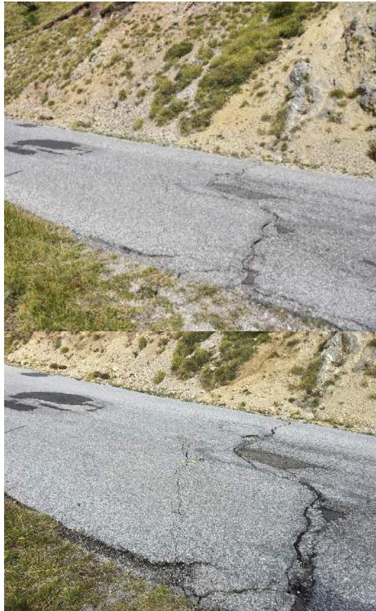
Fig. 19 - Evidence for afterslip at the Forca di Presta road. Above, reactivation of a pre-existing asphalt crack with virtually no displacement and a very thin new oblique crack, as observed on August 27; below, downwarping on the left side (west) and widening of the oblique crack (4 to 5 cm downthrow); new cracks have also appeared in the ground on both sides of the road (photograph taken on August 31).
